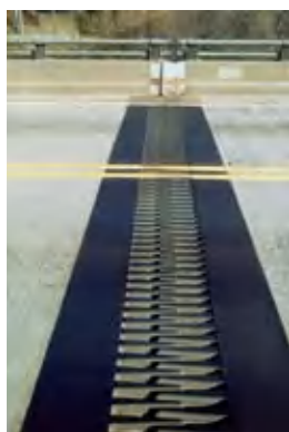
An open expansion joint on a bridge
